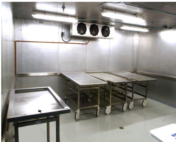
Walk-in refrigeration unit
