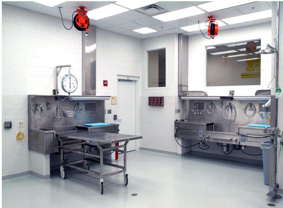
A total of four autopsy work stations with mobile tables
