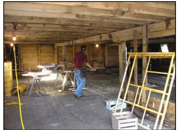
The former stables have been transformed into a temporary workshop for the restoration crew
