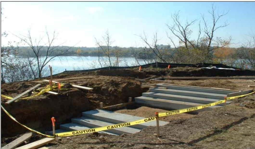
Looking west over Ford Lake, steps leading to the future overlook off the main Segment L1 trail. Construction and landscaping to be completed spring 2005.
