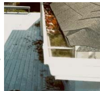
Clogged rain gutters
